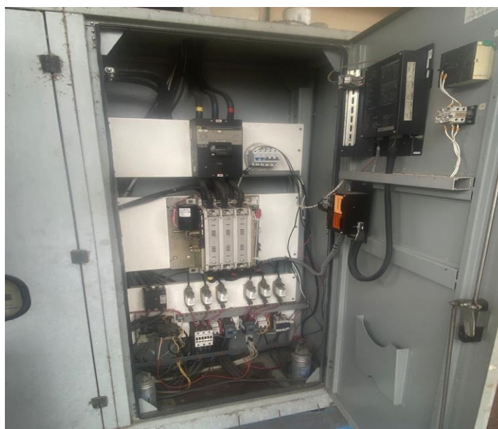
Figura 8. Panel de control, bombas sumergibles
